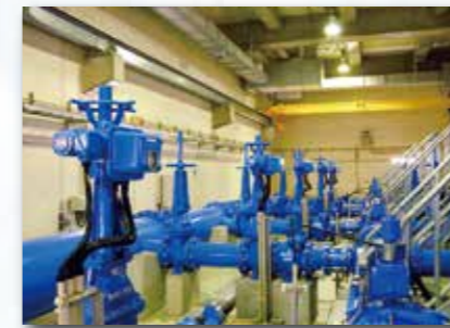
Sewage treatment plant
