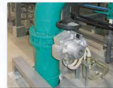
General factory equipment
