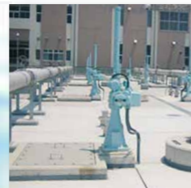
Water purification plant
